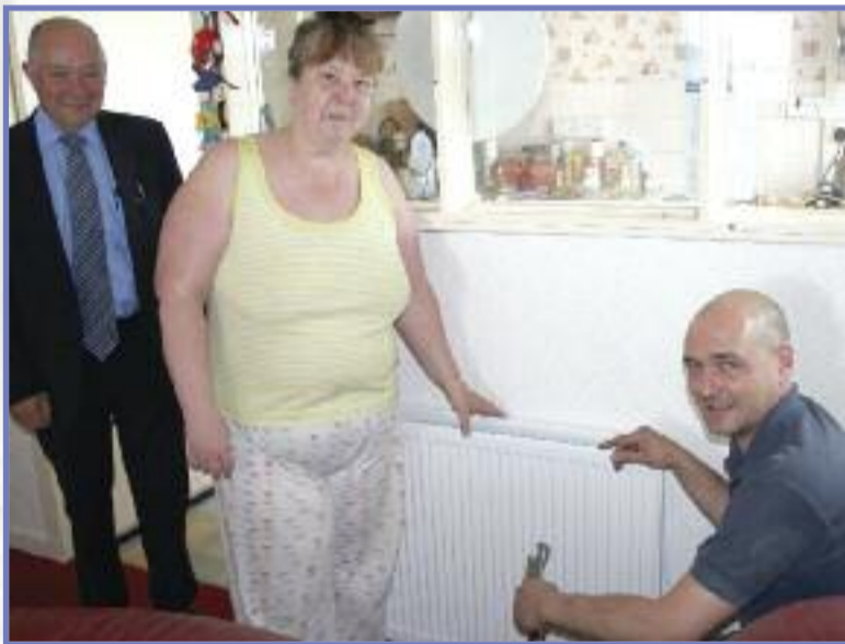
Tenant, Christine McGregor pictured with Robert McKinnon of North Glasgow HA and Davie Smith of City Technical Services during the refurbishment of her flat in Eccles Street
